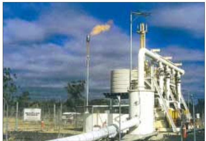
Methane extraction system at Central Colliery coal mine, German Creek. Photo courtesy of NSW Minerals Council
